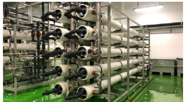
Reverse Osmosis (RO) Water Treatment Plants
